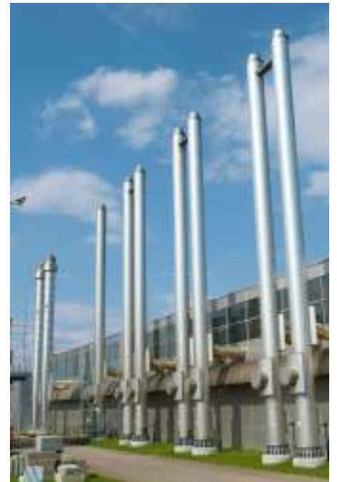
Cogeneration unit on the Airport campus
