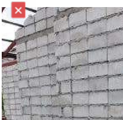
Placement not in a running bond
