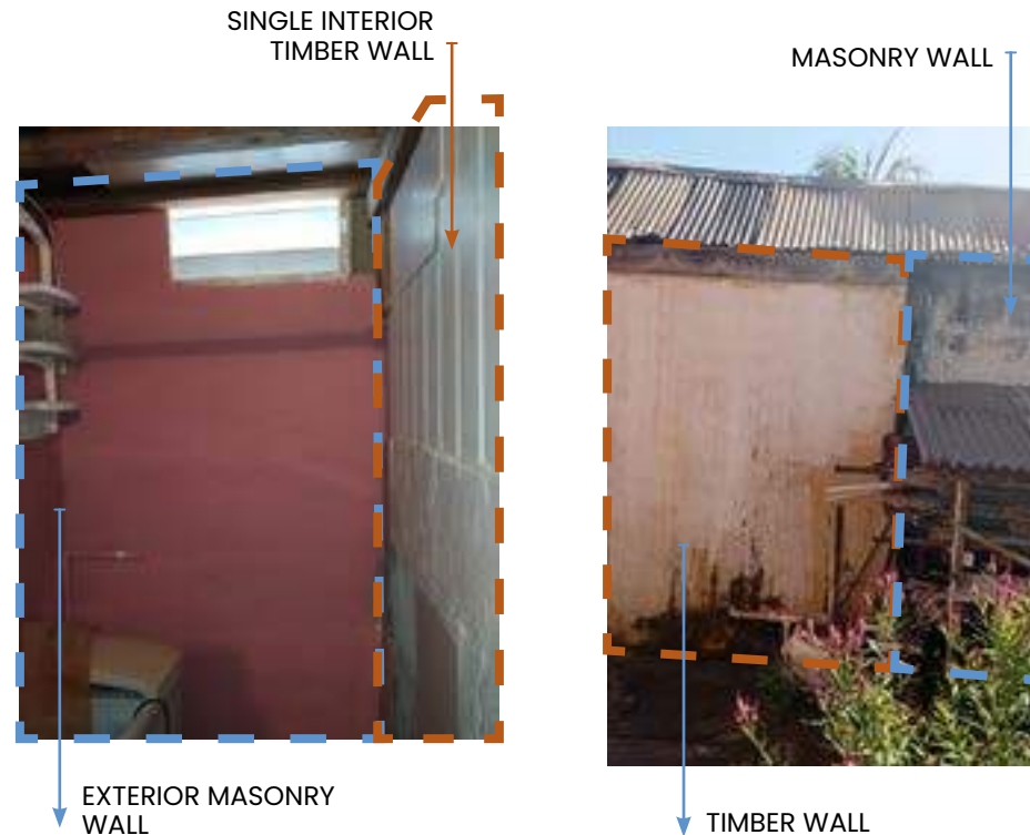
Examples of unstable masonry walls due to adjacent timber walls
